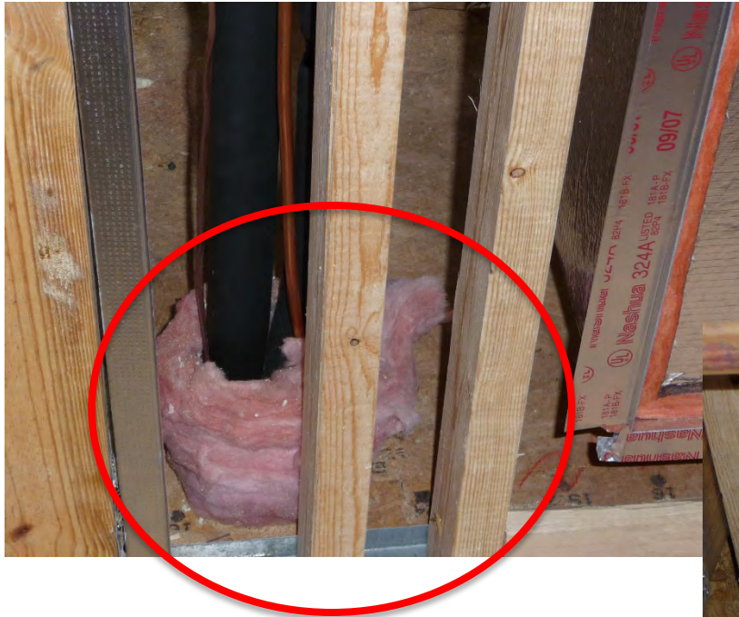
Return Duct Leaks Into Floor Cavity
